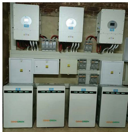
▼ South Africa 40kWh/24KW
